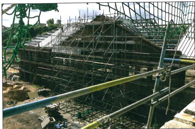
Part of the superstructure taking shape. Completion of the new 'supersurgery' is expected in late March.
