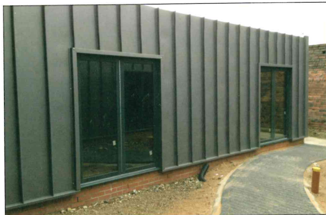
The consulting pods at ground floor level have sheet metal and glazing forming the walls.
