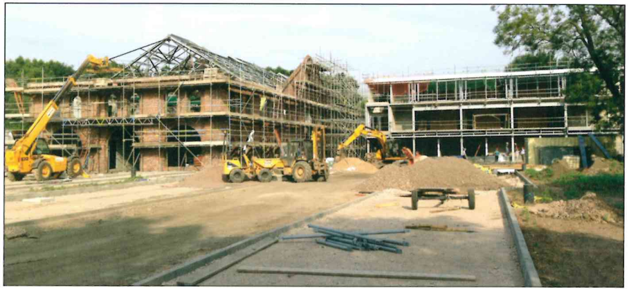
The development combines conversion of the interior of the existing 19th-century foundry (left of picture) with entirely new-build accommodation.
